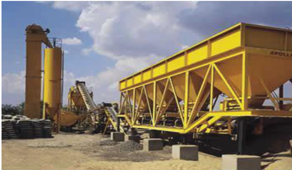
Fig-A5: Computer Controlled Bins for Mixing
